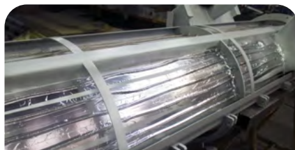
Jacket steam piping
