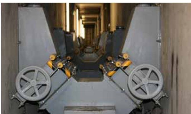
Valves under cells
