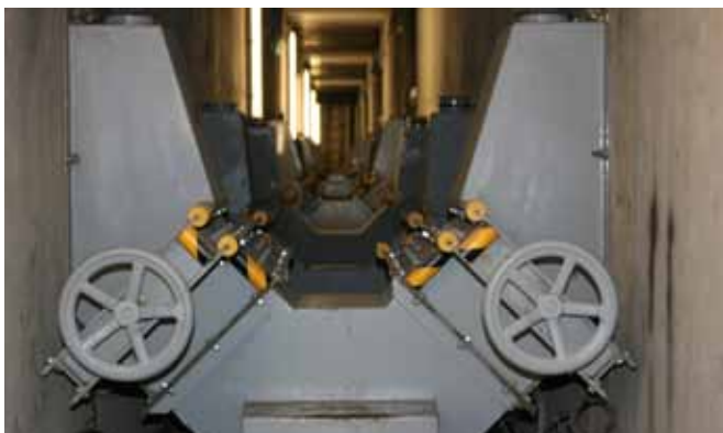
Valves under cells
