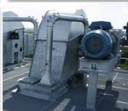
Elevators with discharge suction intakes
