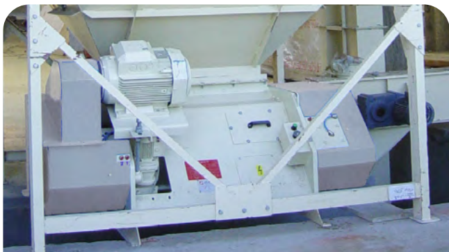
Crumbler beneath cooler
