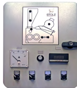
Control cabinet for adjustment of cylinder gap
